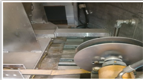
Inside the trailer at front, plow stops on the plow making contact with the plow stops welded to the inside of the front wall
