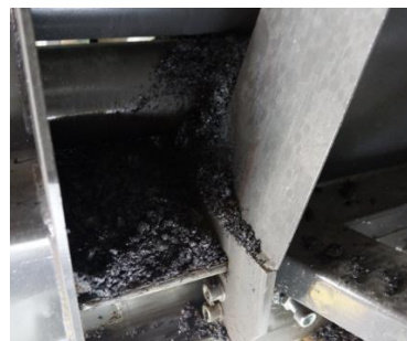
Fig. 66: Asphalt deposits on the slide rail
